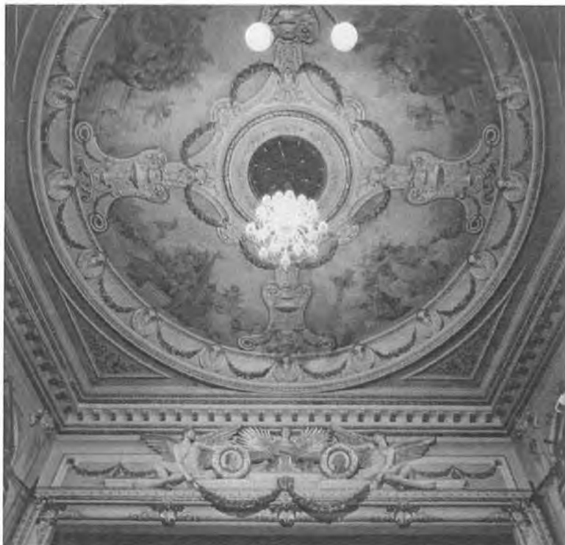
Plate 25 Wyndham's Theatre, London c.1898 one of the many period fibrous plaster ceilings Photo courtesy of English Heritage in Mortars Renders & Plasters (2012) p.109
