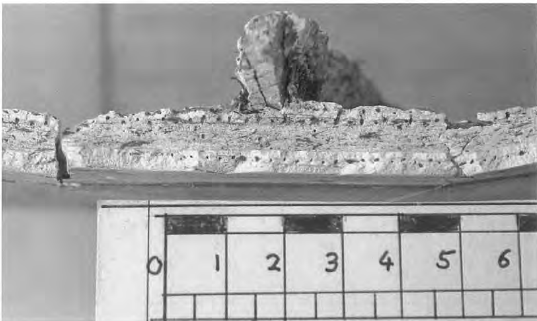
Plate 11 Detail of Plate 10 (above) giving edge on view of plaster section showing exposed hessian scrim incorporated in plaster and lath on edge for additional panel support and with whiter 'firsts' layer distinct from the subsequent greyer 'seconds' layer of plaster
