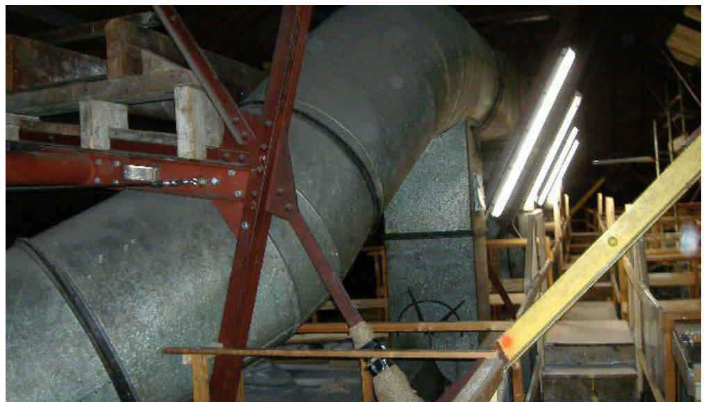
Figure 31: In ceiling voids bulky mechanical plant and boarded walkways (lower right) obscure the fibrous plaster ceiling below and impede its inspection.
